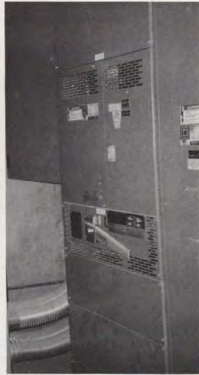
This is the power source for the school.
